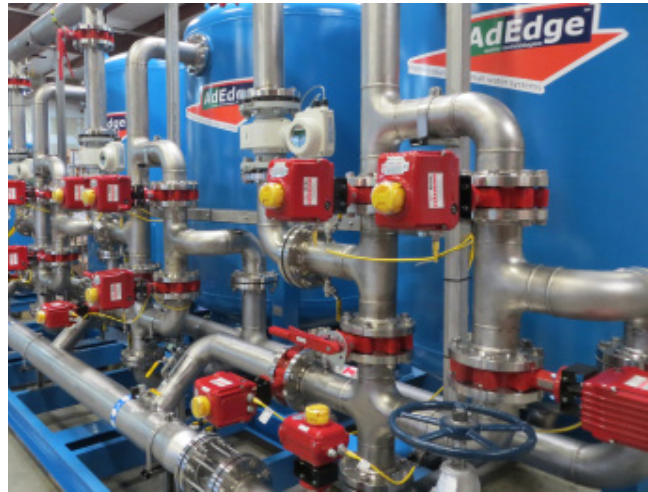
600 gpm manganese removal system in North Carolina using AdEdge's AD26 oxidation/filtration media.
