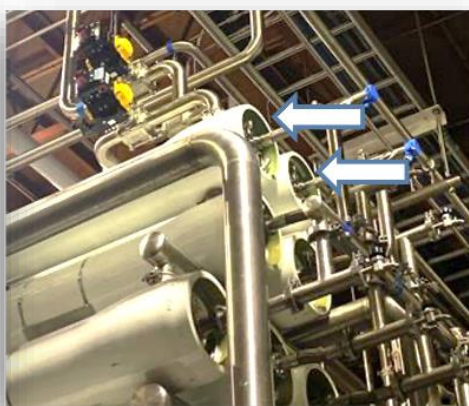
Retrofit of the Reverse Osmosis system with the Flow Reversal technology.
