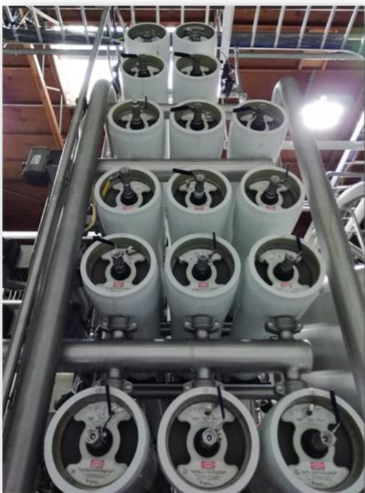
A view of the complete retrofitted RO system designed to optimize the recovery rate.
