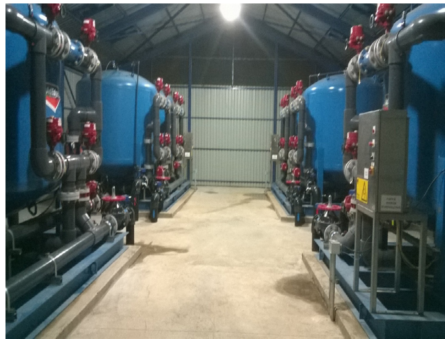
2.7 MGD arsenic removal system in Santiago, Chile using AdEdge's Bayoxide E33 adsorption media.
