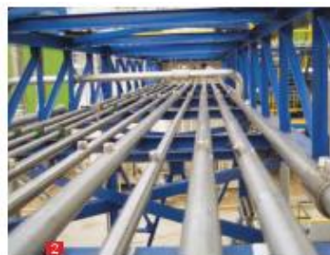
1-2: Vacuum insulated line in industry
