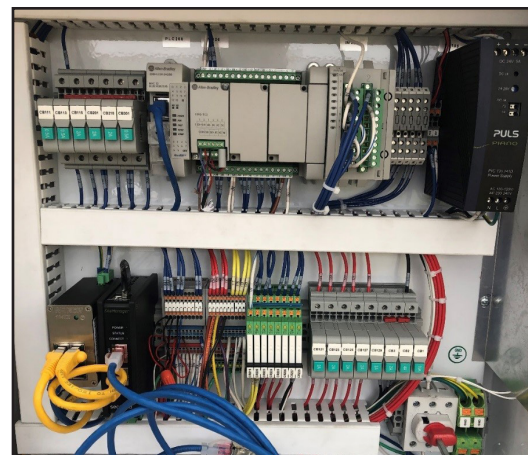
Figure 2. Allen Bradley Control Panel
