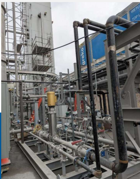
Cold box and Brazed Aluminum Heat Exchanger (BAHX) integration
