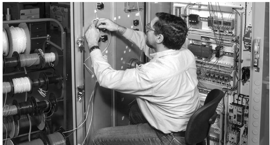
In-house assembly of control panel with PLC and operator interface terminal.
