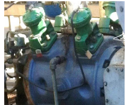
A refinery customer experienced problems with gas leakage from their OEM old style diaphragm unloader actuators
