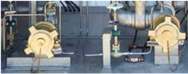
Fill/Drain and Vapor Return
