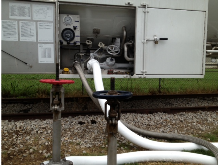
Typical cryogenic piping. Off-loading liquid ethylene from a DOT-113C120W Tank Car.
