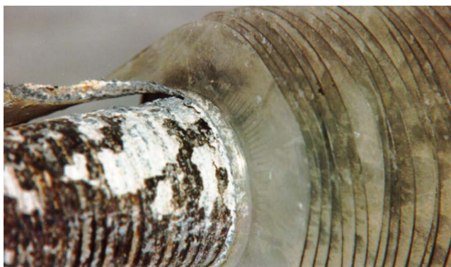
▲ Figure 13. If the condition of tubes and fins is significantly degraded due to corrosion, the bundle will need to be retubed.
