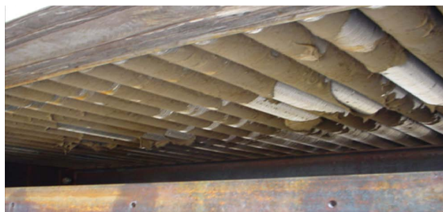
▲ Figure 6. Finned tubes can become fouled. Make sure they are inspected for fouling during visual inspection of air-cooled heat exchangers.
