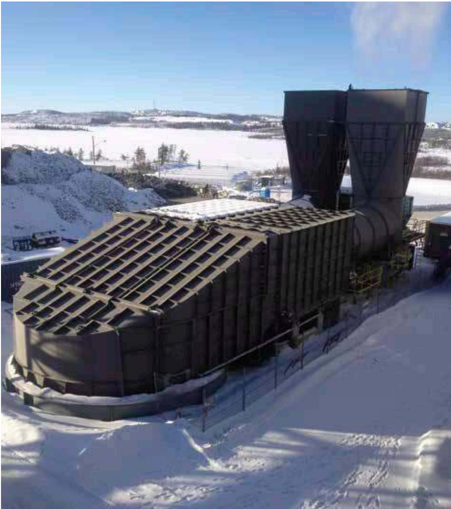
Ventilation air needs to be responsive to working temperatures as well as specific activities.
