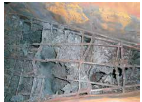
Basket damaged by fire in an Air Preheater.
