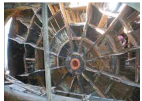
Rotor damaged by fire in an Air Preheater.
