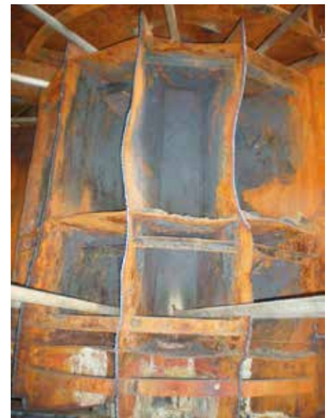
Rotor damaged by fire in an Air Preheater.
