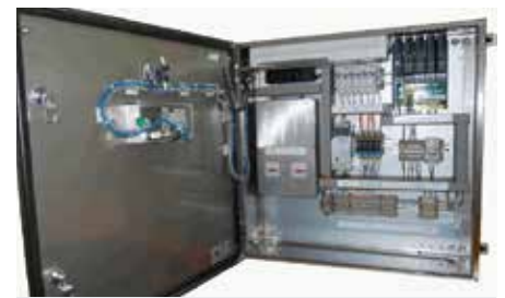
Fire detection monitoring equipment.
