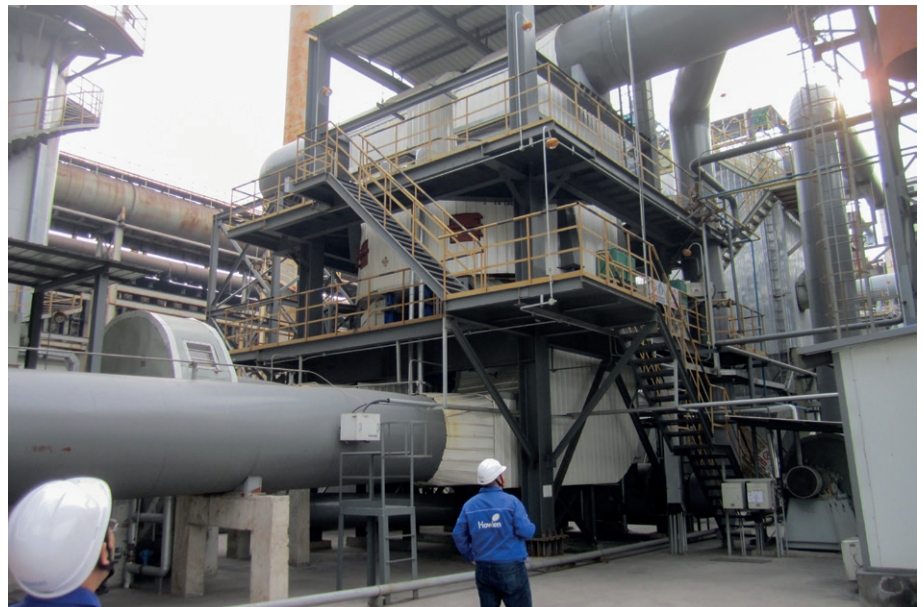
Figure 4: Coal gas charging GGHS operating.
