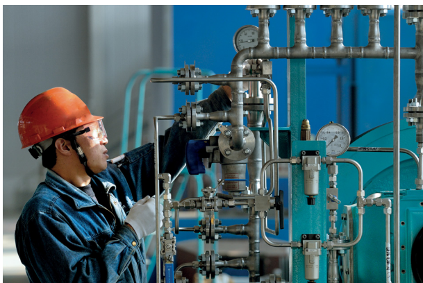
Figure 3. Global service team working on a compressor.
