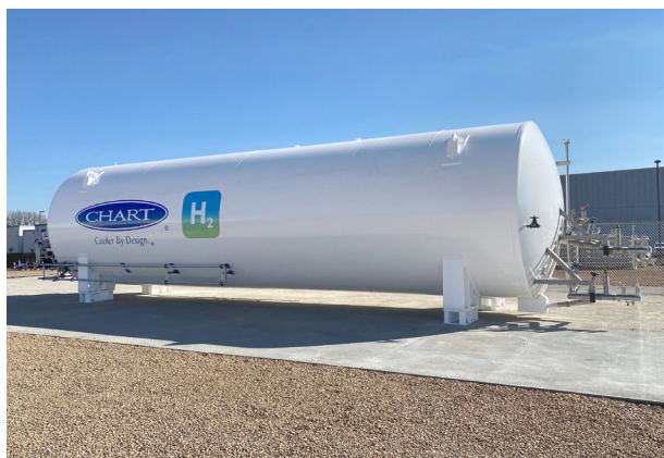
Figure 2. A Chart hydrogen tank at the storage stage of the hydrogen value chain.
