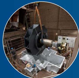
Waste gas fan assembly within a steel sinter plant
