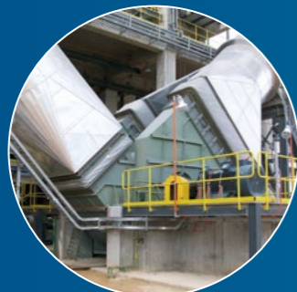
Induced draft fan in a cement plant
