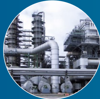
Fans within an oil refining process
