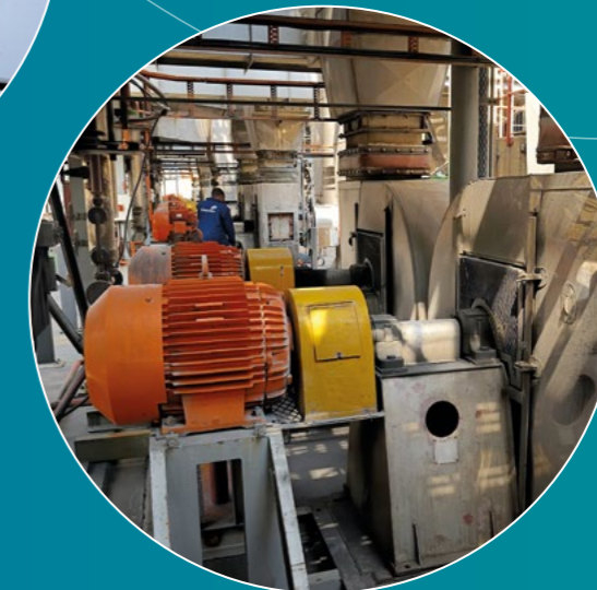
Fans in operation in a brewery
