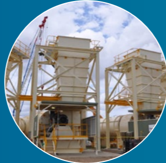
Main ventilation fans for underground mine
