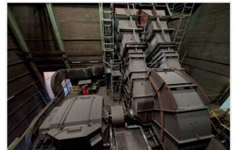
The original waste gas fan in situ.
