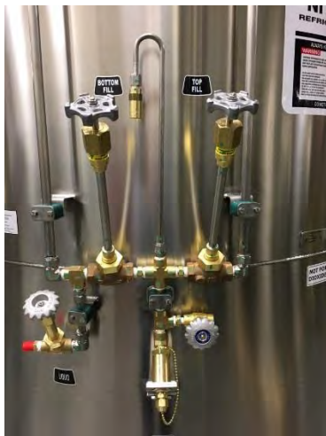
Current Top/Bottom Fill Manifold
