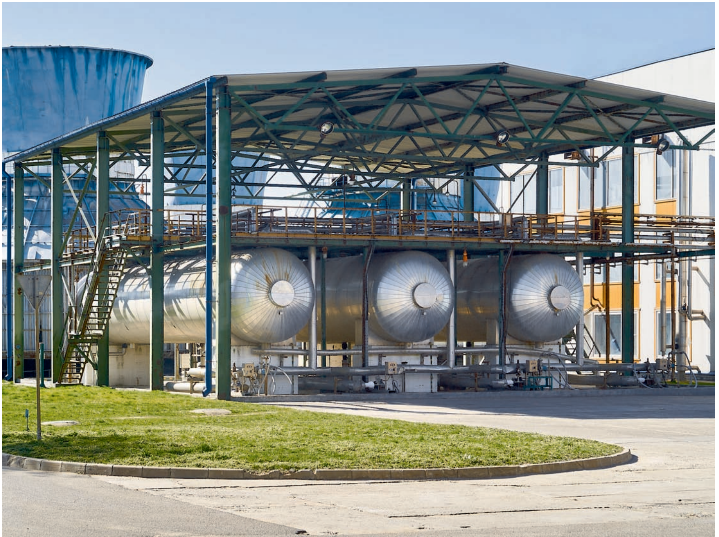
Cryogenic liquid CO 2 storage tanks
