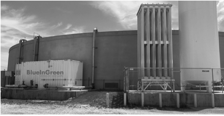
Figure 1: Increase Capacity without Disrupting Operations. The side-stream dissolution process of the SDOX® solution enabled Mountaire Farms to retrofit significant treatment capacity to overloaded treatment basins without disrupting operations. The side-stream process draws influent up-and over the basin wall into the SDOX® system and then returns the supersaturated solution back to the basin.
