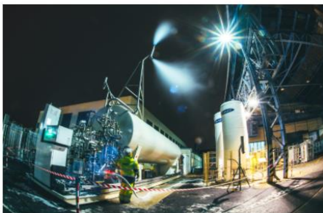
LNG Fueling Station during FAT
