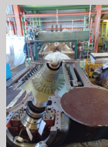
Air compressor, Major Overhaul
