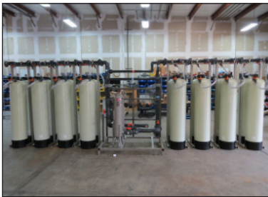
MODULAR TREATMENT SYSTEMS
