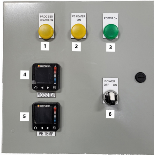
Figure 23 - Low Voltage Panel for TBC (Exterior)
