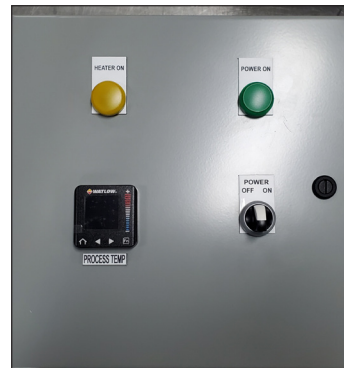
Figure 17 - Low Voltage Panel (Exterior)
