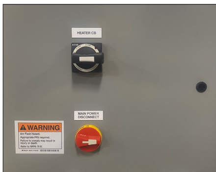
Figure 15 - High Voltage Panel (Exterior)
