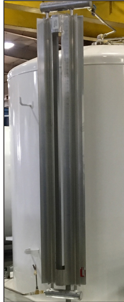
Figure 28 - Pressure Build (PB) Vaporizer
