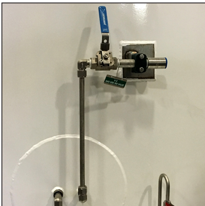
Figure 32 - Gas Use Valve (V-2)
