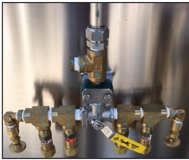
Figure 10 - Safety Relief Valves with Diverter Valve
