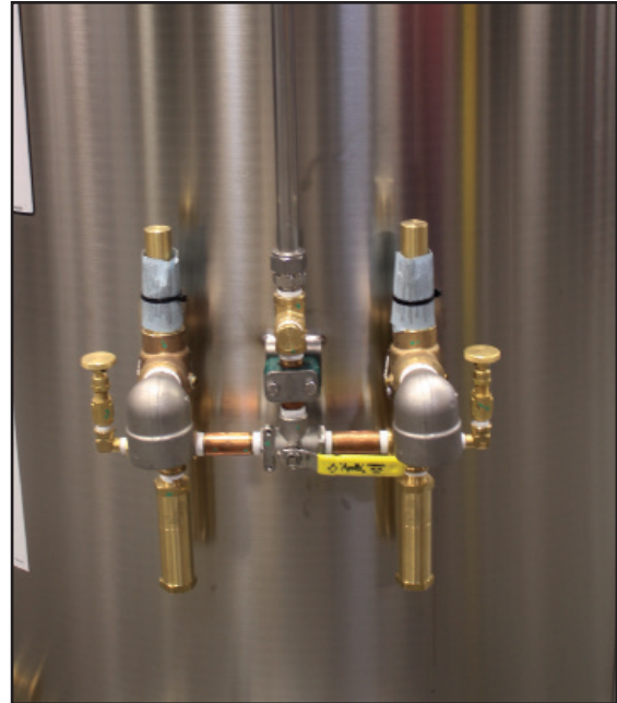
Figure 20 - Diverter valve, Bleed-off valve, Primary Relief valve (top) and Secondary Relief valve (bottom)
