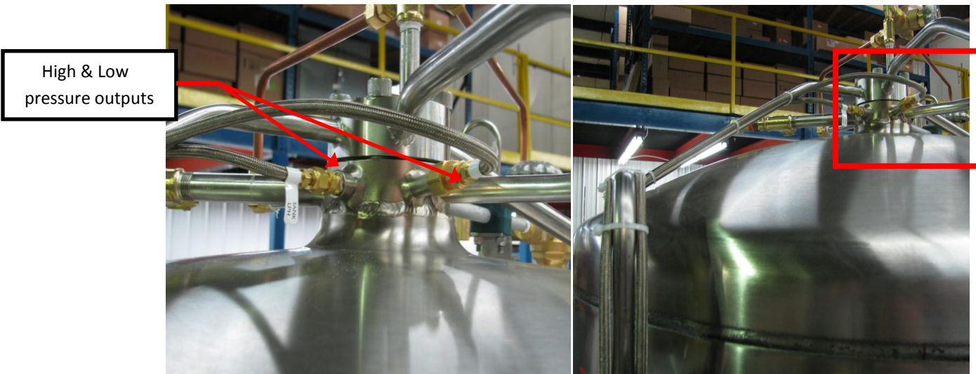
Figure 3.1.3-7: High and low pressure lines connected to high and low pressure outputs of the tank.
