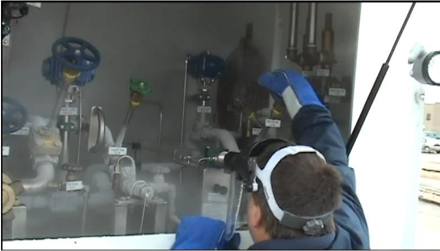
Figure 78 – open Manual Vent Valve V-05, close V-05 at less than 25 psig
