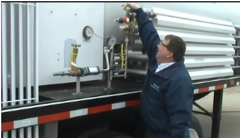
Figure 44 – close Gas Use Isolation V-25
