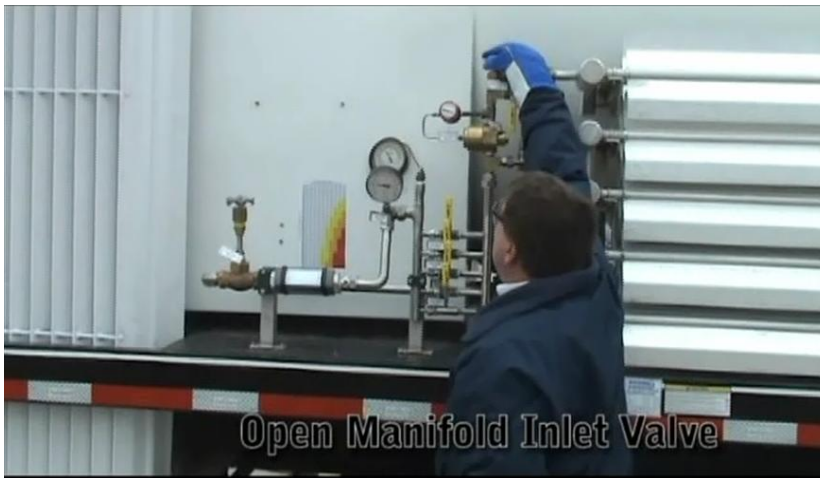
Figure 33 - Open Manifold Inlet Valve
