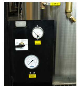
Lower Mounted Controls
