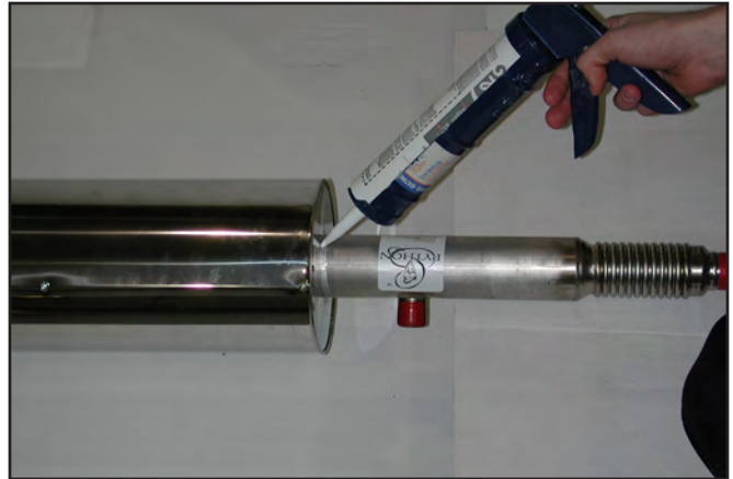
10. Caulk all edges with silicone sealer. (Sides and seams where metal cover overlaps itself.)
