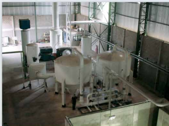
Steel Mill in Brazil ASV77200 (2,029 Nm 3 /hr) Plant
