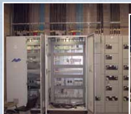
Control Panel and Motor Control Center
