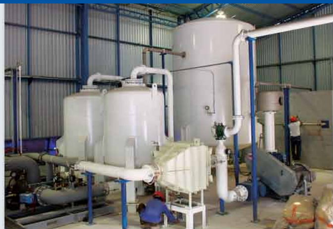
Steel Mill in El Salvador ASV14500 (381 Nm 3 /hr) Plant
