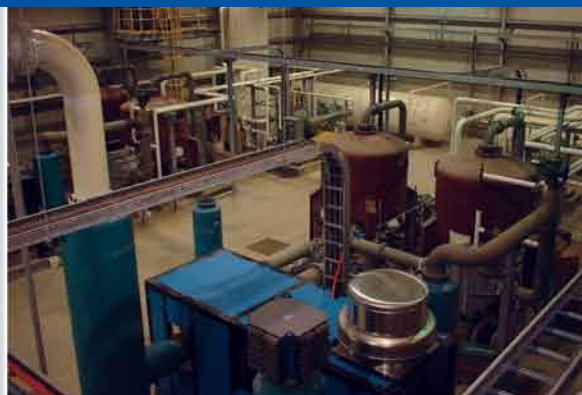
Uranium Mine in Canada Two ASV24500 (644 Nm 3 /hr) Plants
