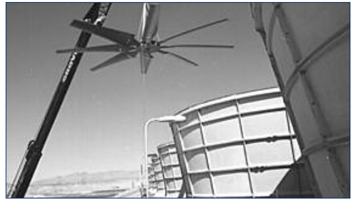
Typical Large Cooling Tower Fan with VR Stack Fig. 9
