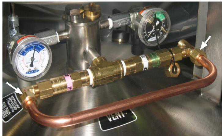
Pressure relief vent tube assembly on CO 2 storage vessel. (Arrows indicate compression fitting connection.)
