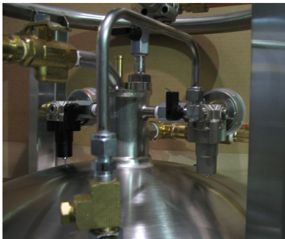
SMC style regulator plumbed into the pressure building circuit viewed from the "liquid side" of the circuit.
