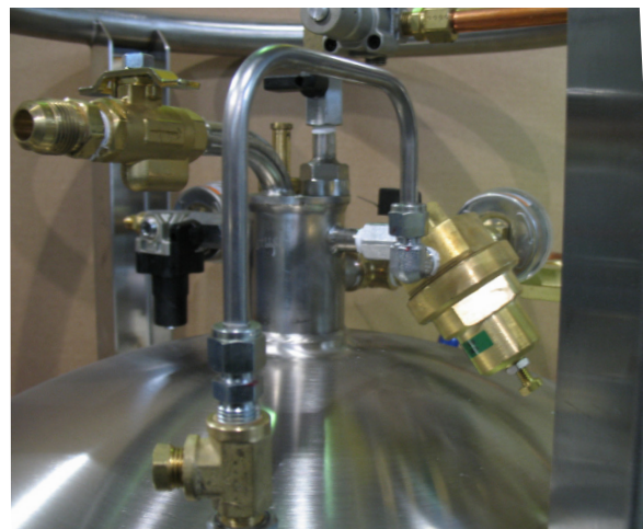
Rego style regulator plumbed into the pressure building circuit viewed from the "liquid side" of the circuit.
