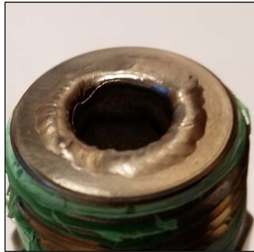
Crack in welded joint example
