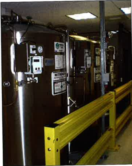
Two 1,500 liter nitrogen Perma-Cyls supply liquid nitrogen to Genzyme's Low-loss fill system. One 1,000-liter Perma-Cyl supplies nitrogen in gas phase throughout their building.
