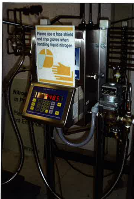
Low-Loss fill station controls. Middlesex installed this system at Genzyme to help curb excessive dewar handling.
