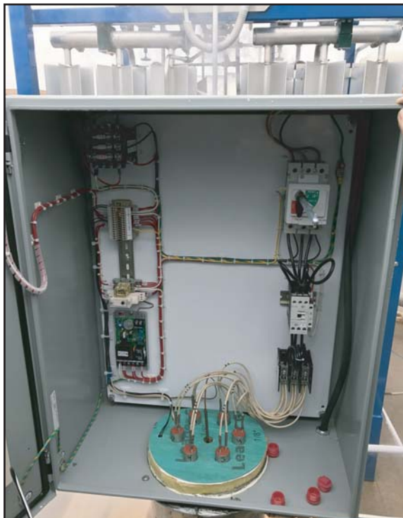
Inside of Thermax Electric PB Vaporizer
