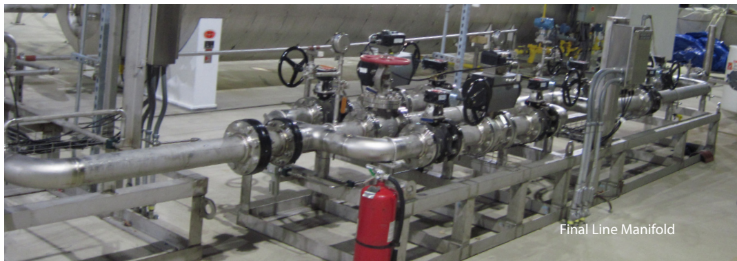
3 tanks, vaporizer, IFWB and manifolds
