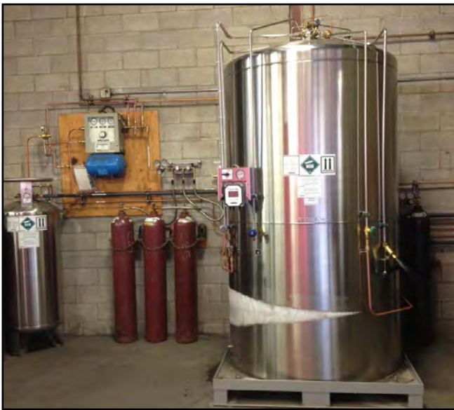
Indoor Installation of a Perma-Cyl 3000HP tank
