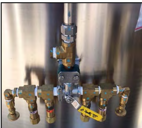
Figure 9 - Safety Relief Valves with Diverter Valve
