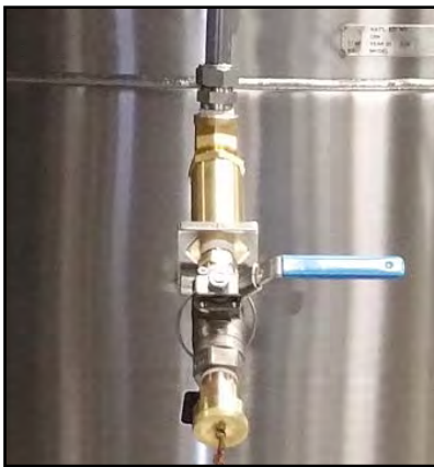
Figure 3 - Fill Isolation Valve
