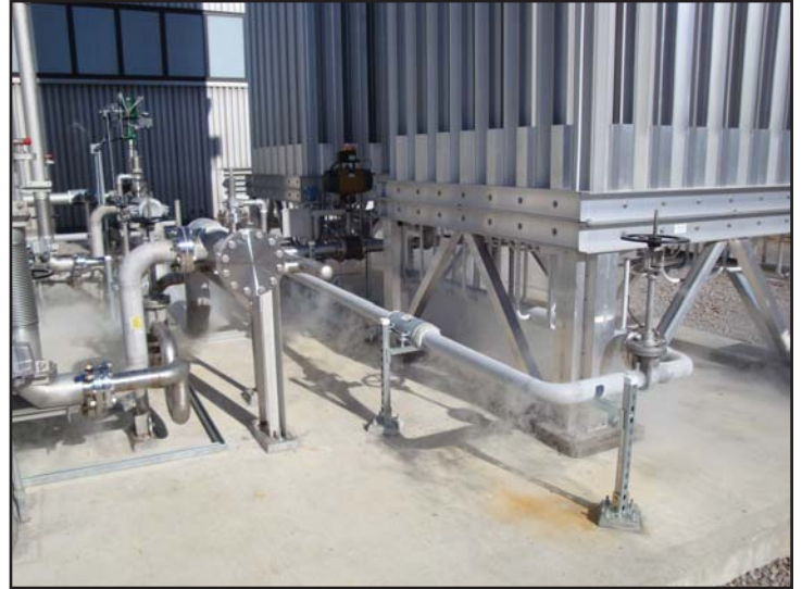
LN 2 High Pressure Tank Supply System
