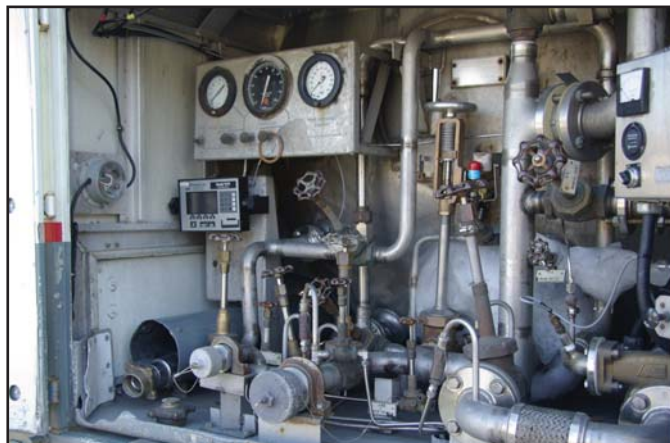
Typical cryogenic tanker plumbing with traditional turbine flow meter system.
