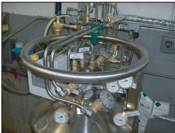
Argon Maximizer Plumbing
