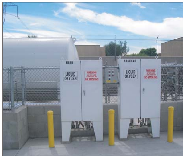
Liquid Oxygen - Main & Reserve Remote Fill Cabinets
