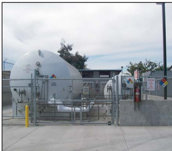
Bulk Medical Gas Installation - Main & Reserve Storage Tanks
