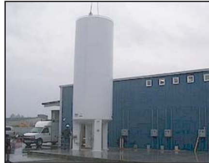
VS-Siphon 100 Tank in Argon Service
